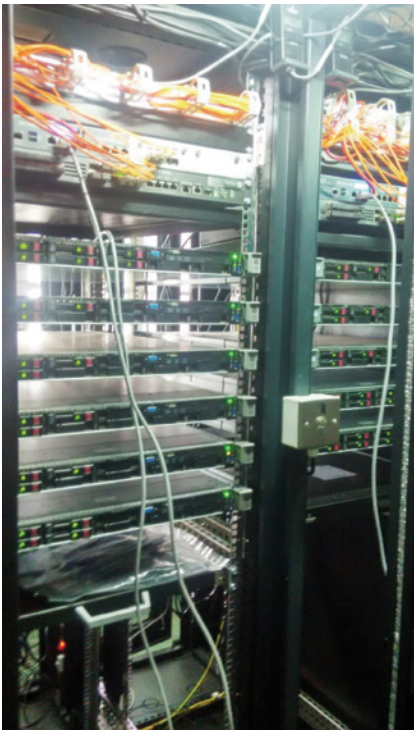
Fig: Server Room: Windows stack and Linux Stack
