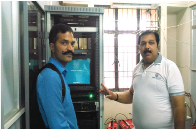
Server Room, Aranya Sadan, Lucknow
